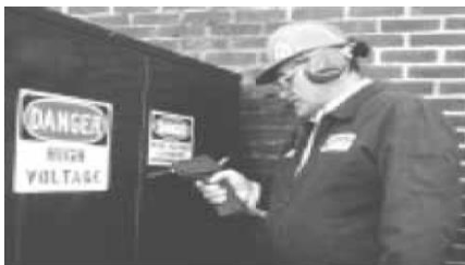
Test switchgear, transformers, etc. for arcing, tracking & corona.
