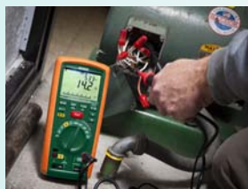
Insulation test on pump motor
